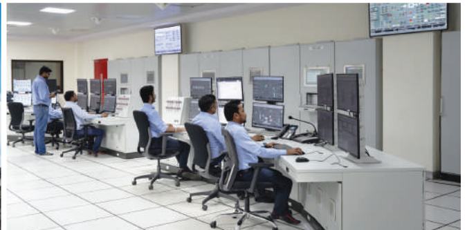
Main Control Room
