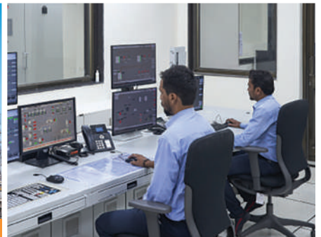
Water Control Room
