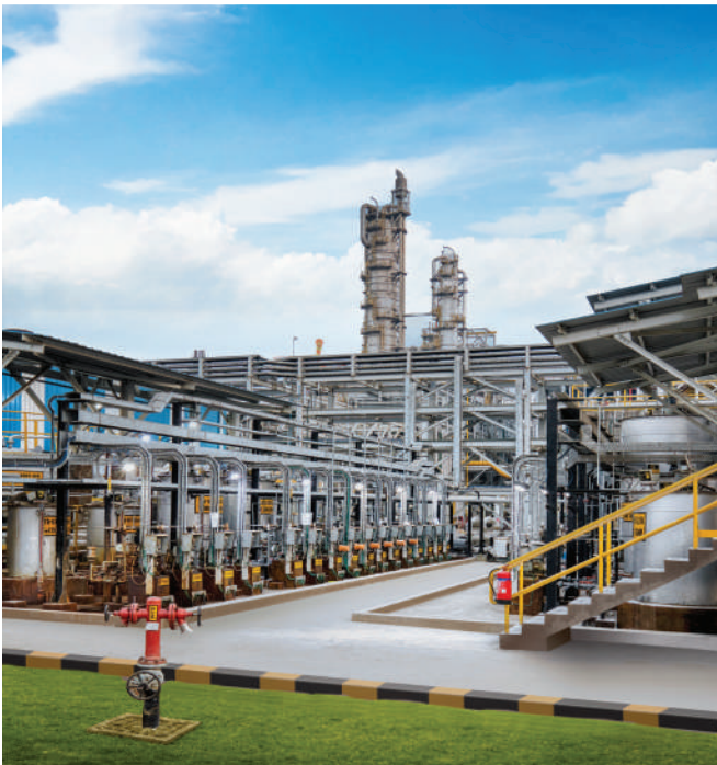
Reverse Osmosis (RO) Plant
