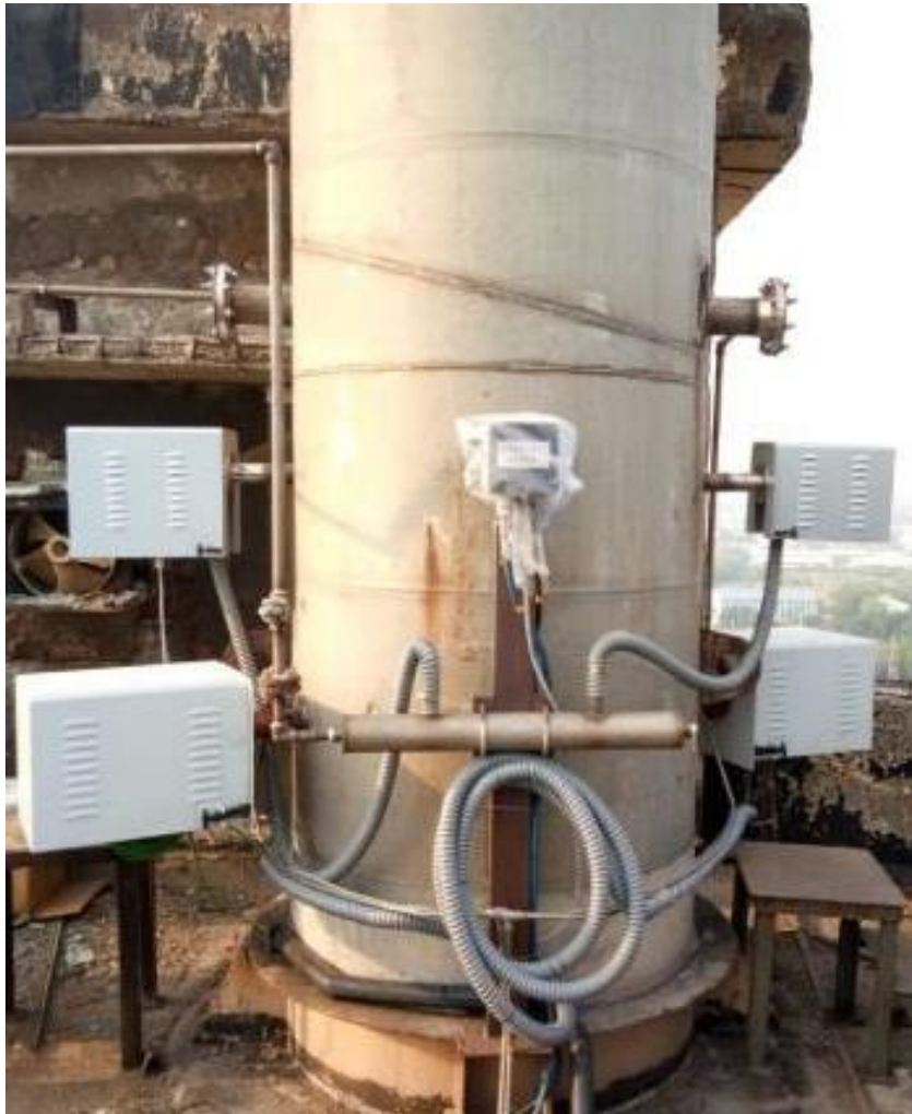
NPK-1&2 Stack at K-1
