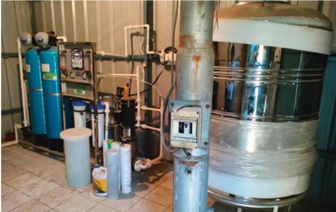
RO unit installed at Kanpoli, Dahej for clean water for all
