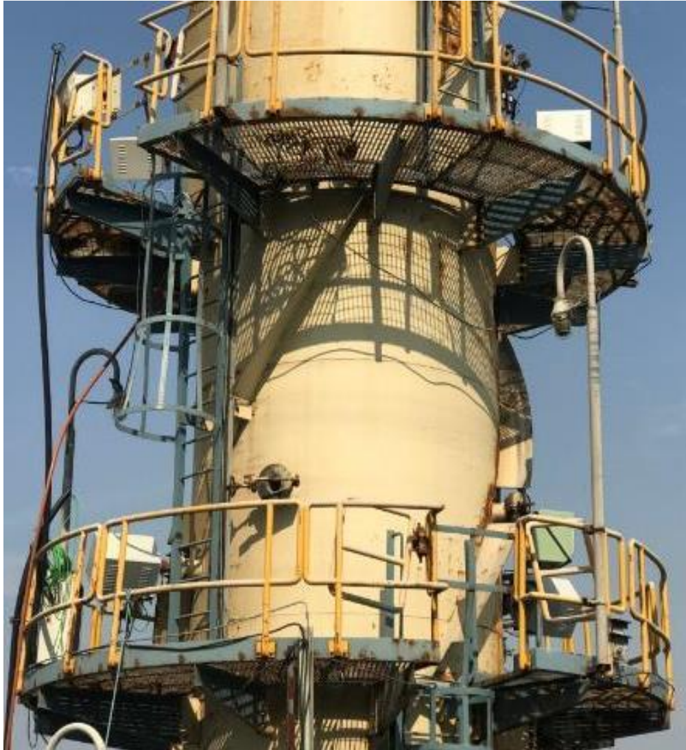
NPK-1 Stack at K-1
