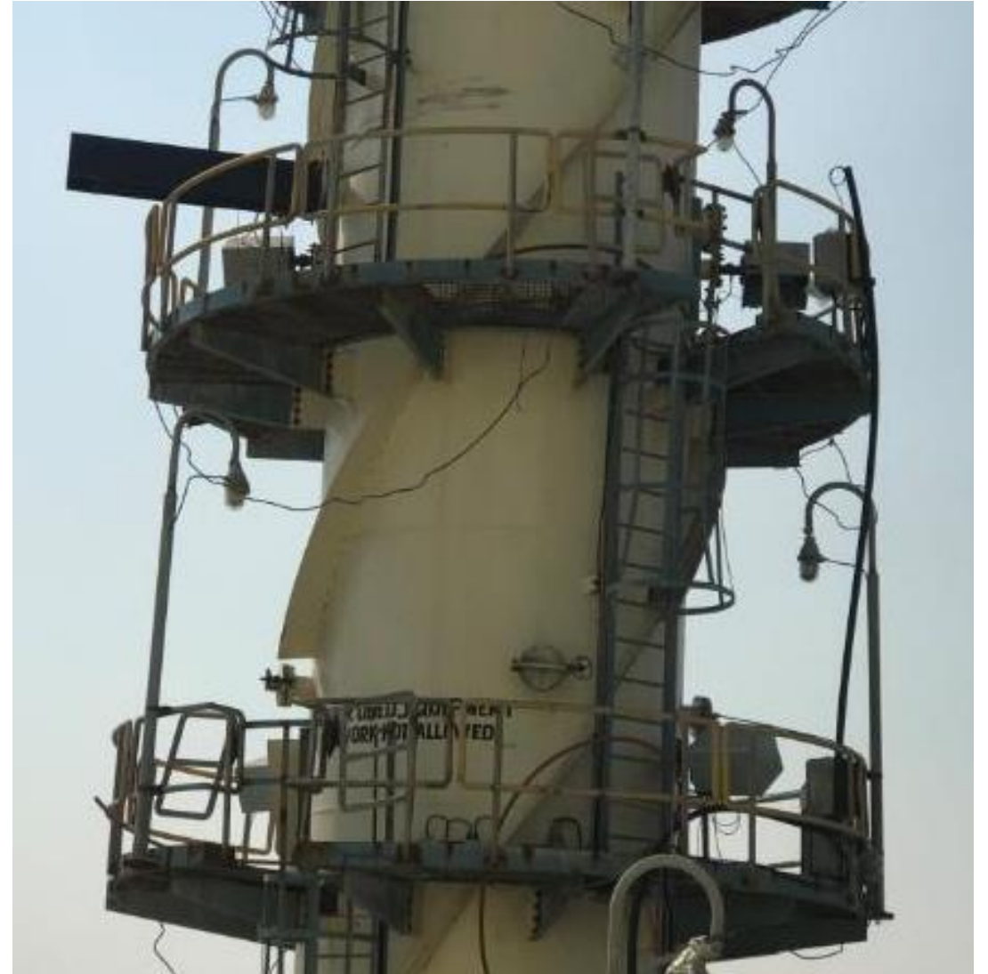
NPK-2 Stack at K-1
