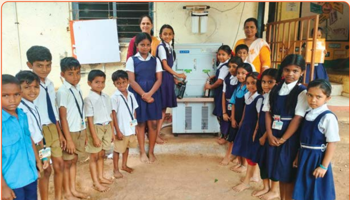
Safe drinking water facility being provided for school children to ensure their good health and well-being
