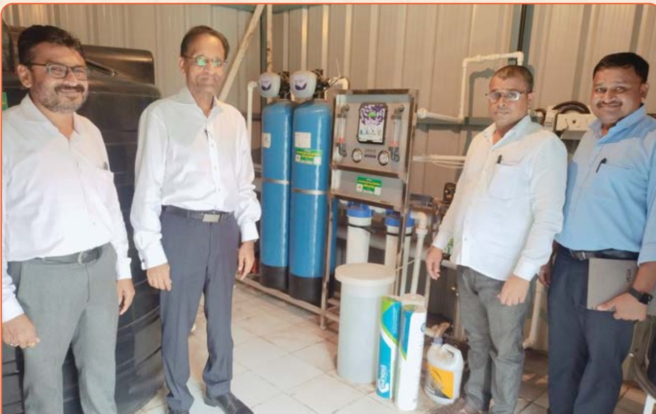
Installation of 1,000 LPH RO unit to provide safe drinking water to the community
