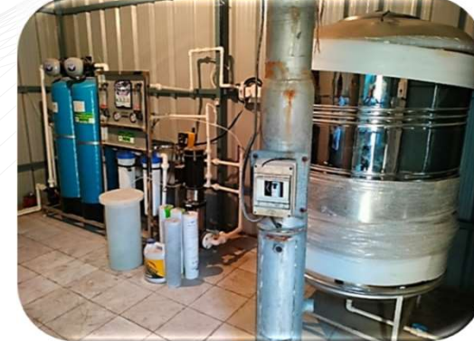
Project- Social Welfare RO Drinking water facility, Talaja
